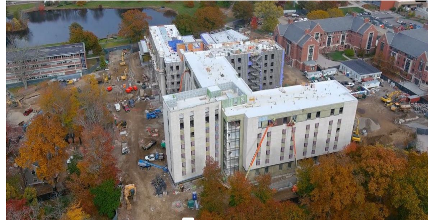
View looking southwest of construction on the two L-shaped wings of the Residence Hall
