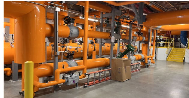
SUP Interior View of 125 psi Steam Header
